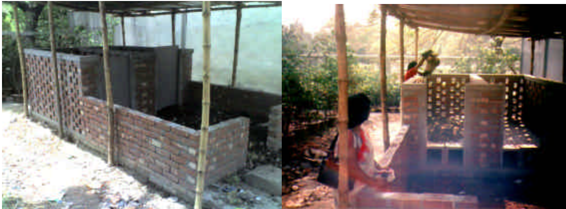
Front view of the compost facility constructed in the premises of the National Nursery Consortium located at Kalabagan, Dhaka
