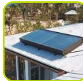
Roof top solar panel
