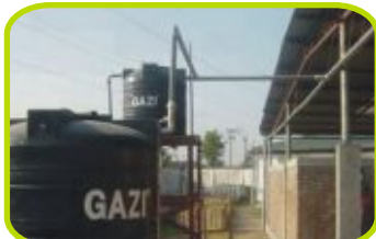
Rain water harvesting system
