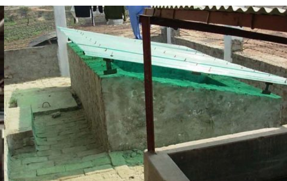
Leachate treatment tank
