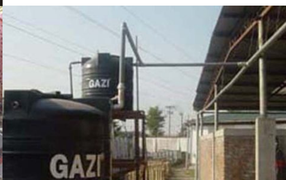
Rain water harvesting system
