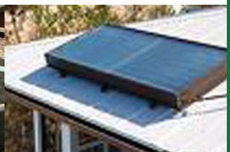
Rooftop solar panel
